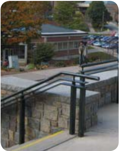
Exterior Stair Handrail
